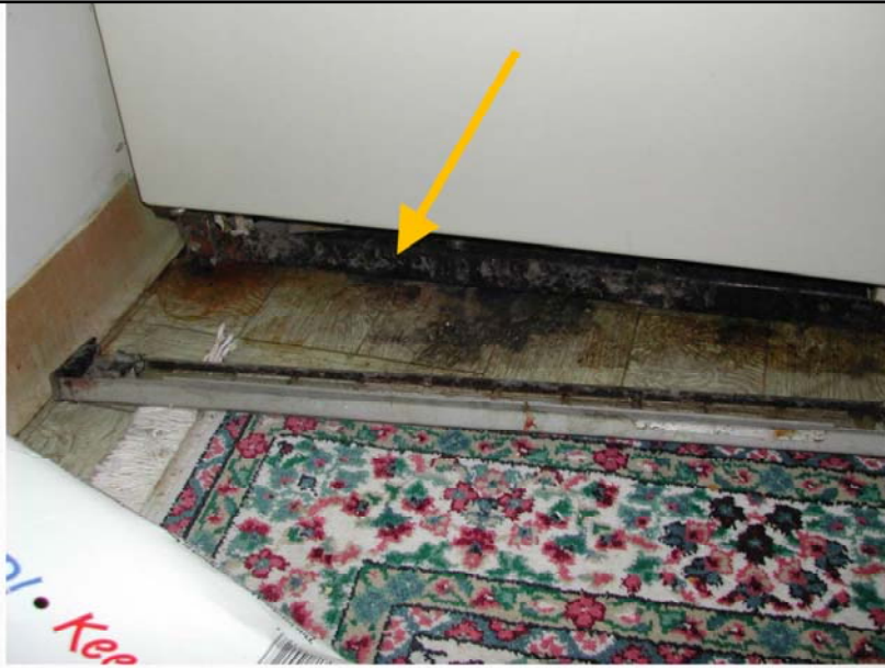
Leaky refrigerator drip pan causes mold
