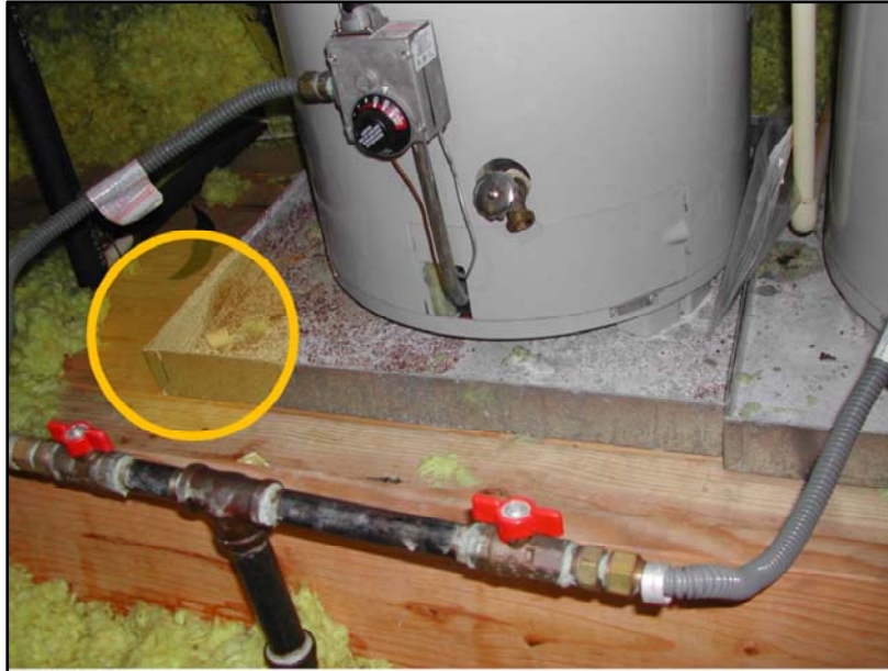
Drain pan in the event of heater leak
