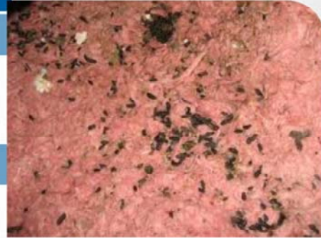
Rat feces in insulation
