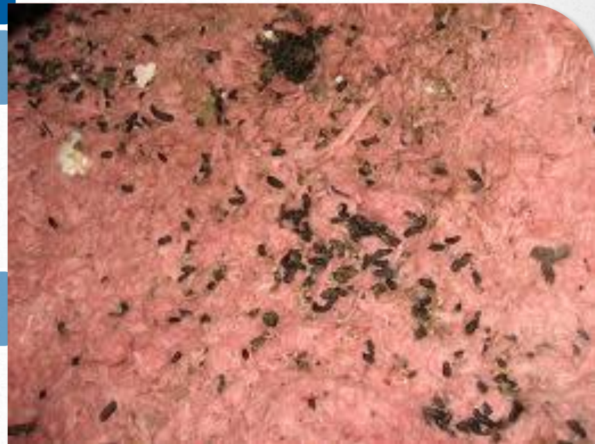
Rat feces in insulation
